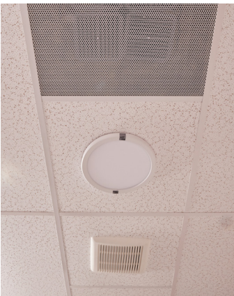
Modern and efficient fixtures
